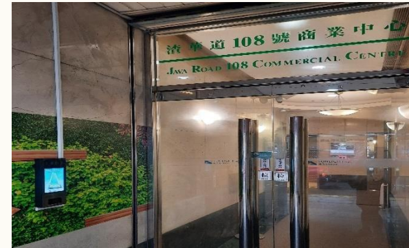
Remote access control system at Java Road 108 Commercial Centre May 2025
